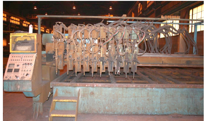
Linde CM350 before retrofit
